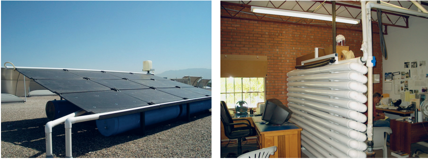
Figures 22–23. The double-play system built at Zomeworks in 2005, with figures depicting the rooftop radiator (figure 22, left) and a PVC water array in the interior of building (figure 23, right). 67
