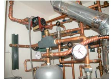
primary loop and plumbing in mechanical closet
