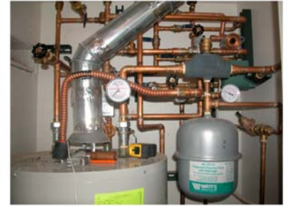
primary loop and plumbing in mechanical closet
