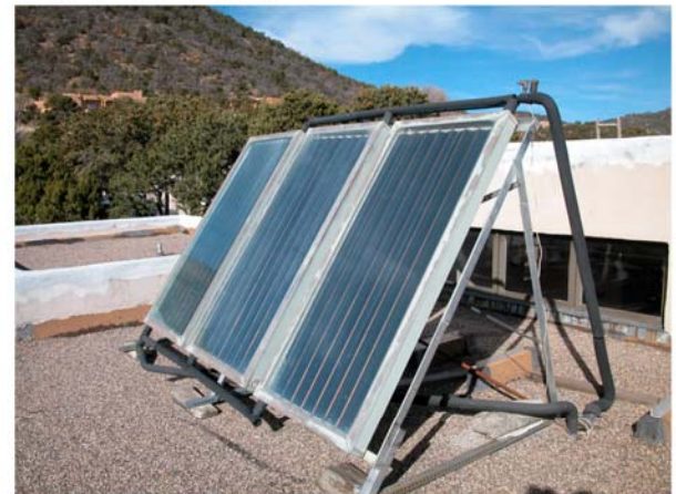
glazed collectors tilted for heat optimization
