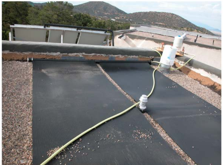
exterior radiators on the roof
