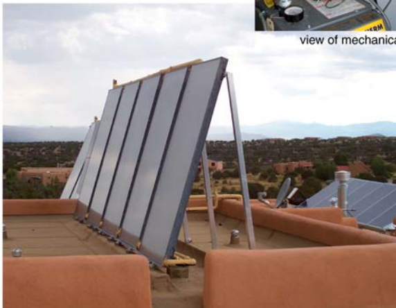
glazed collectors tilted at optimum angle for heating can also be used for cooling
