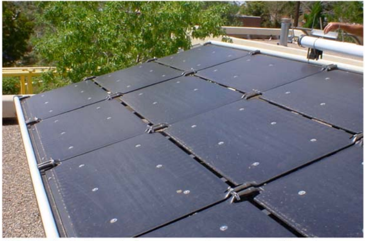
Wetted plastic plate 'sky mat' radiators are mounted on the roof at a slight angle to encourage passive thermosyphoning.
